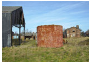
Derelict buildings je021712153.jpg
