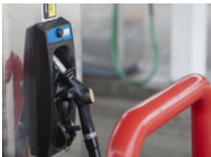
Diesel pump je031220120083.jpg
